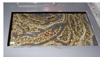
Sludge and oil floating during long shutdowns
